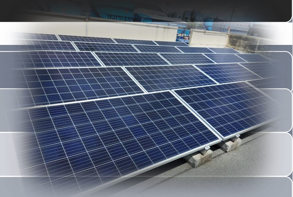
Solar PV Installations at Oil Jetty Port Louis Harbour, Mauritius
